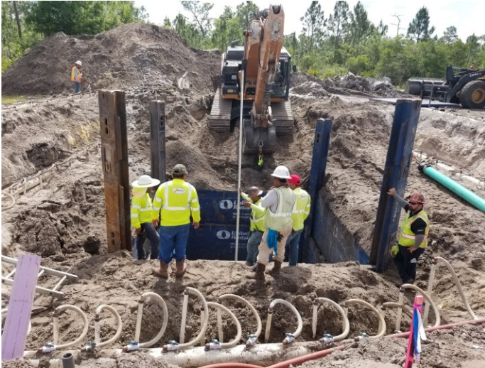
Excavation being done and shoring being installed for new lift station structure.
