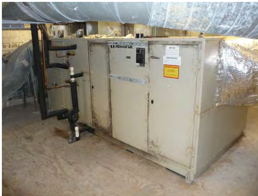
The two Existing custom-built air-handling units at the public safety building will be retrofit with new Temtrol DX cooling coils as part of this scope.
