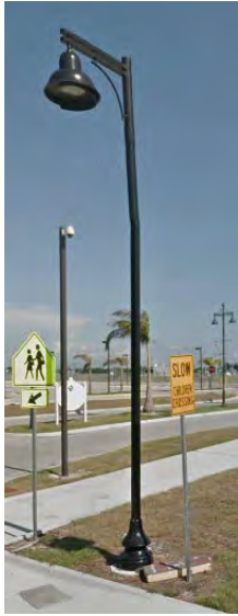
Existing Belltop Fixture - 250W HPS
