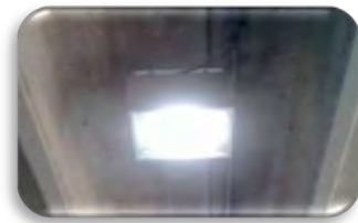
LED Light Fixture
