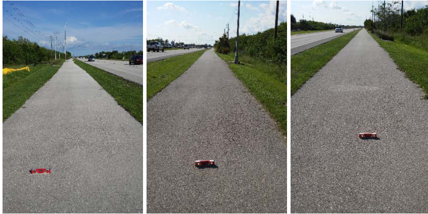
Figure 4-1 – Select locations with non-compliant cross slopes.
