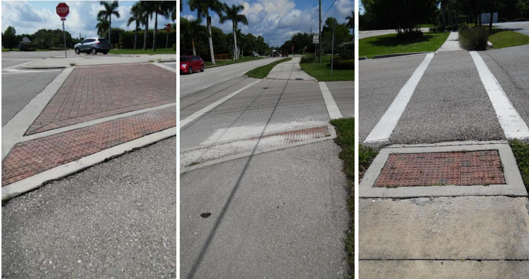
Figure 4-4: Curb ramps with tripping hazards and debris. Map ID's 69, 77, and 90.
