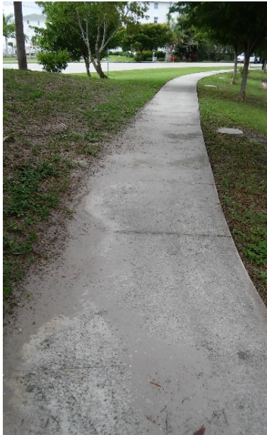
Figure 4-4 – Sediment accumulation along path
