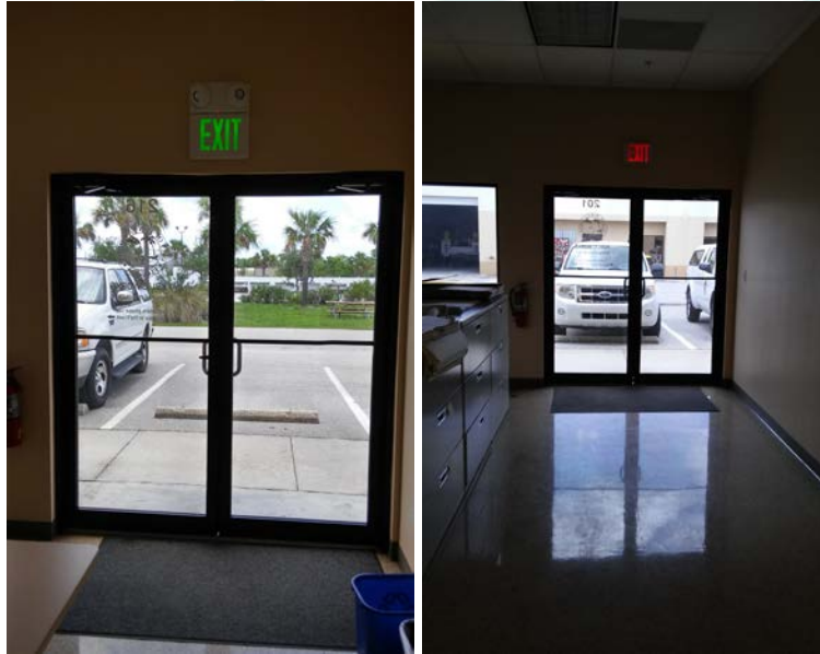
Figure 4-3 – Examples of exit doorways without ADA compliant signage.
