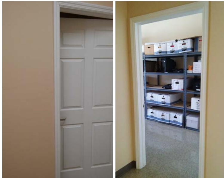
Figure 4-2 – Example of a doorway without ADA compliant signage.
