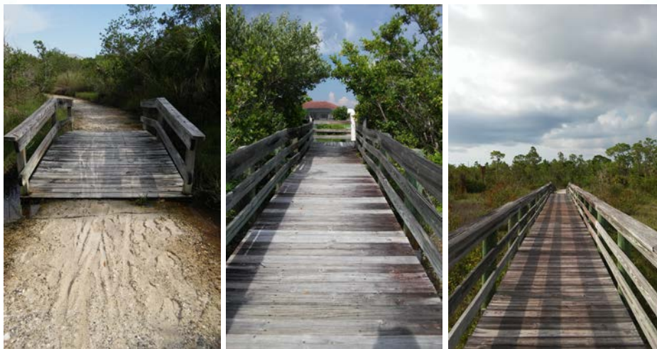
Figure 4-5 – Sediment accumulation along path
