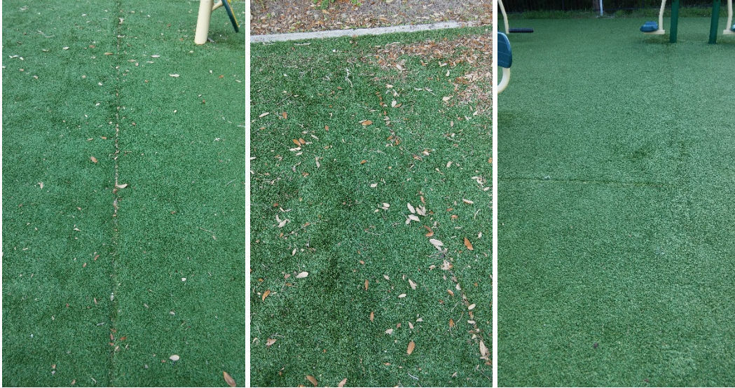
Figure 4-3 – Artificial Turf Tripping Hazards.
