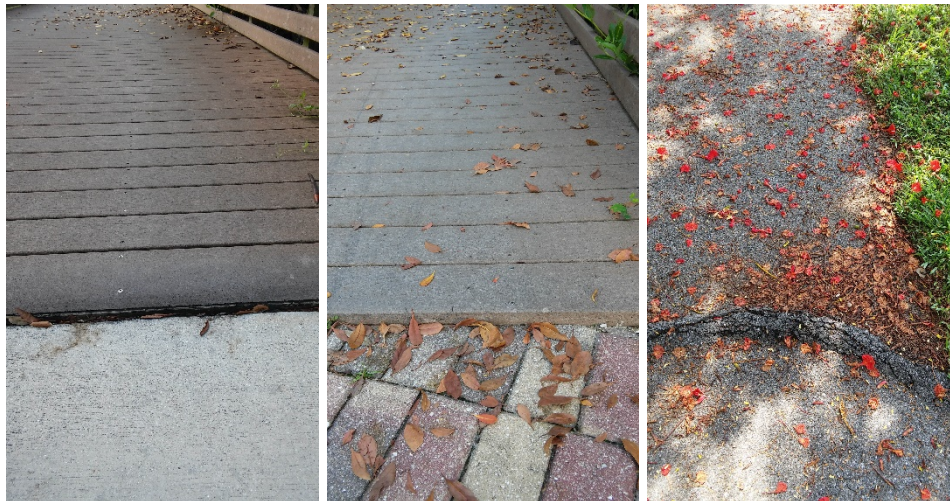
Figure 4-2: Tripping hazards located along pathway.
