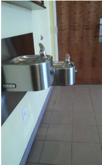
Figure 4-16 –Water Fountains at Restroom
