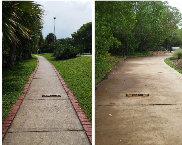
Figure 4-2 – Select locations with non-compliant cross slopes.
