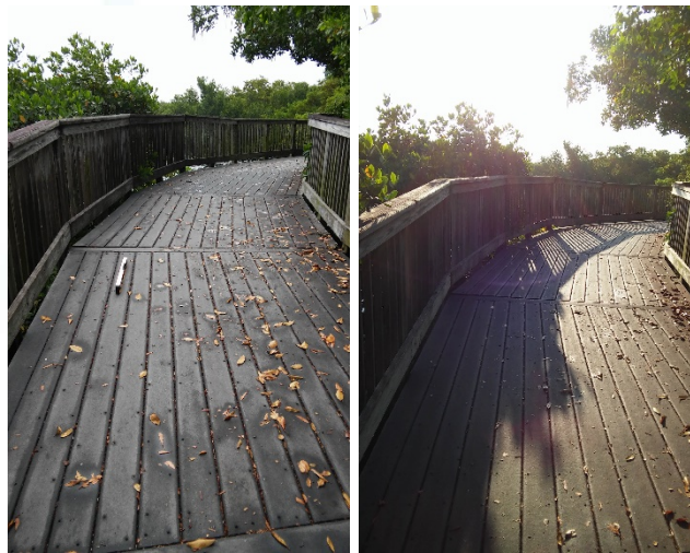
Figure 4-3 – Select locations with non-compliant cross slopes.
