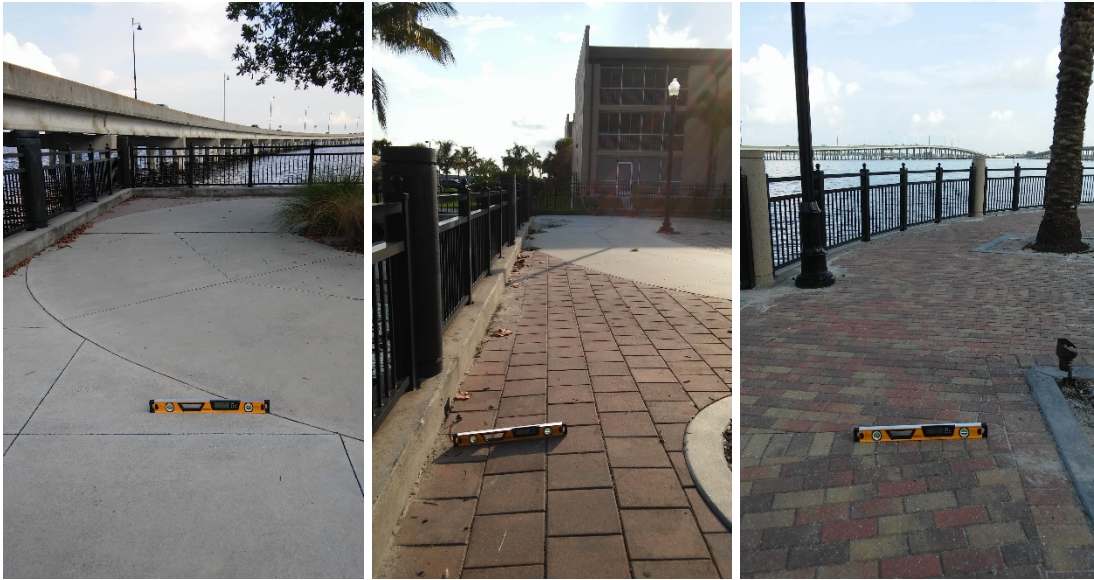
Figure 4-4 – Select locations with non-compliant cross slopes.
