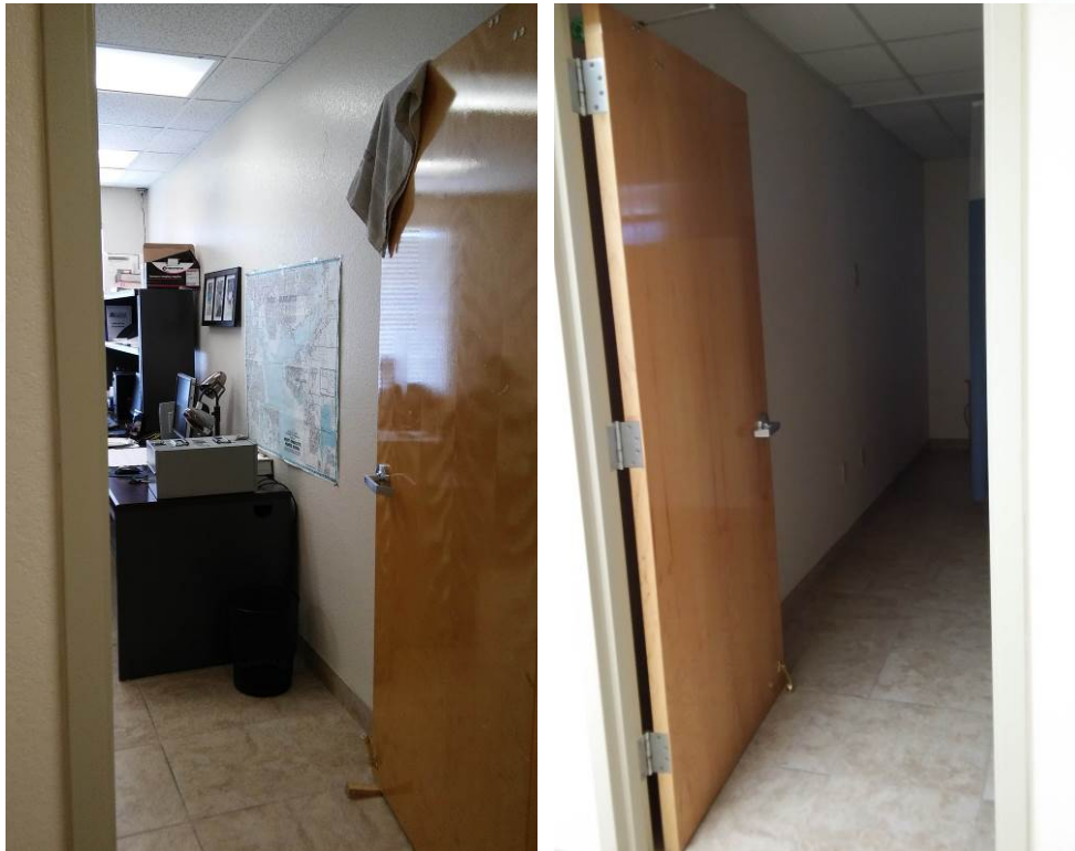
Figure 4-4 - Doorways without signage.=
