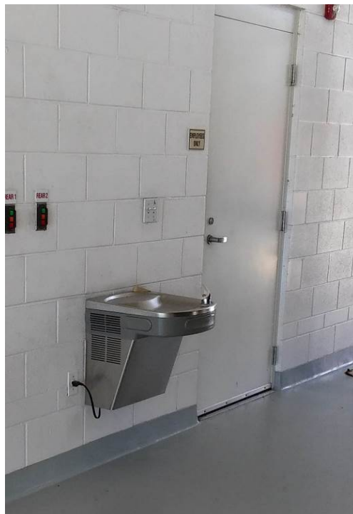
Figure 4-5 - Single Drinking Fountain
