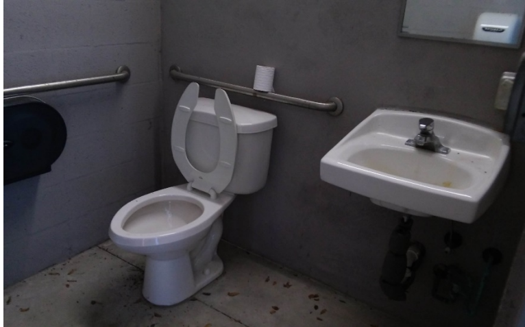
Figure 4-9 – Example of restroom violations
