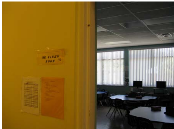
Figure 4-6 - Doorways without ADA compliant signage.
