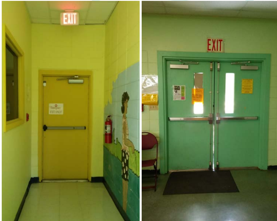
Figure 4-7 – Exit doorways without signage.
