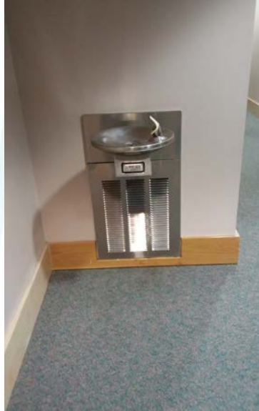
Figure 4-5 – Single Drinking Fountain.
