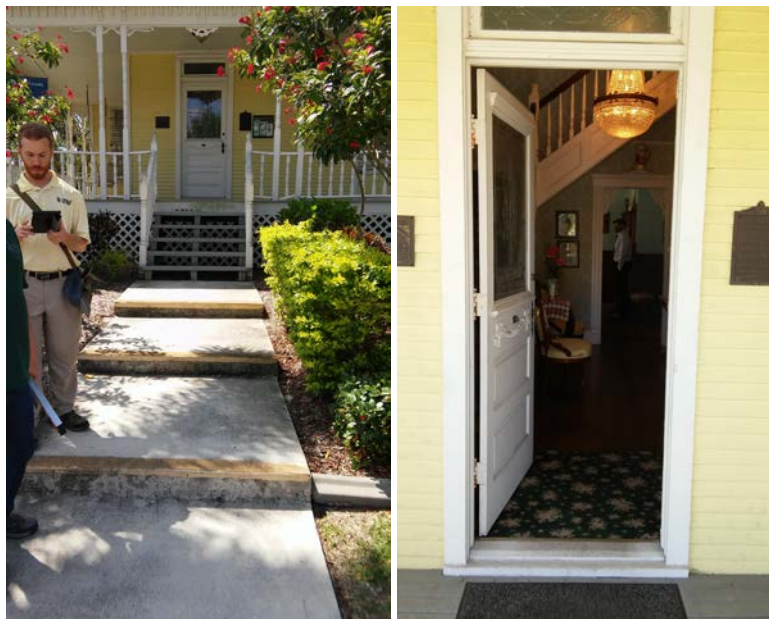
Figure 4-2 – Non-Accessible Front Entrance to Building
