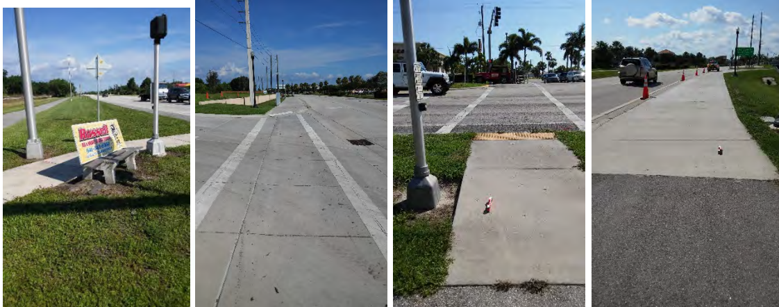
Figure 4-2 – Miscellaneous Barriers to Accessibility along the US-41 Trail
