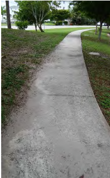
Figure 4-4 – Sediment accumulation along path
