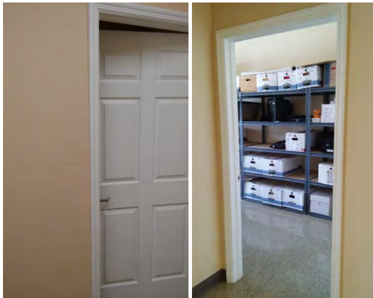
Figure 4-2 – Example of a doorway without ADA compliant signage.
