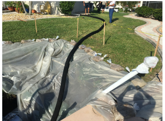
6. DIRECT PLASTIC DRAIN PIPE BEYOND WASHOUT AREA. USE SANDBAGS AND STAKES TO KEEP PIPE IN PLACE.
