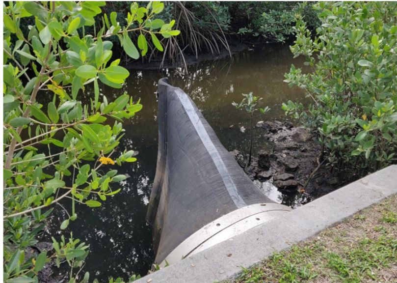
Photograph 4.9 Stormwater Check Valve for Backflow Prevention
