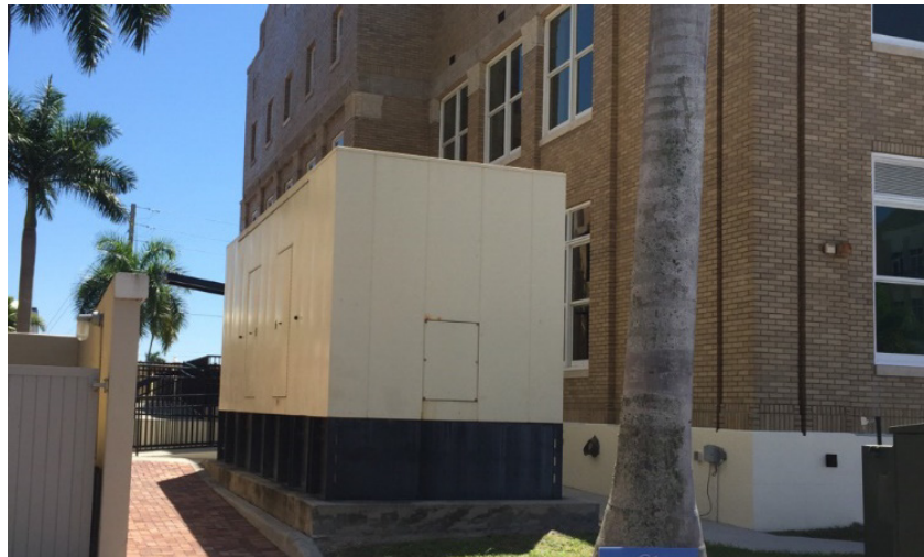
Photograph 4.10 Elevation of Backup Generator at Historic Charlotte County Courthouse
