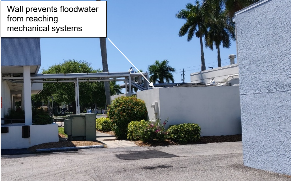
Photograph 4.12 Dry Floodproofed Mechanical Systems at County Tax Collector’s Office
