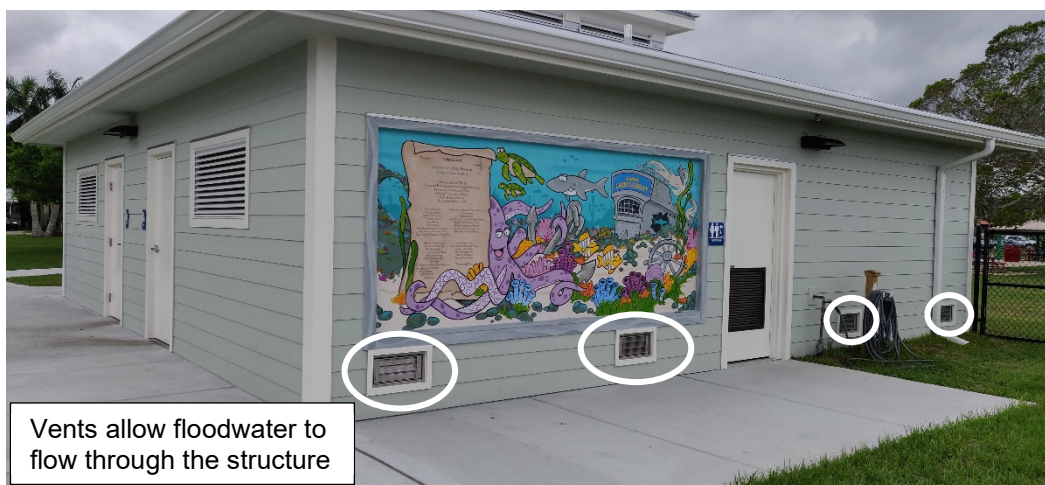
Photograph 4.11 Flood Vents for Wet Floodproofing at Gilchrist Park
