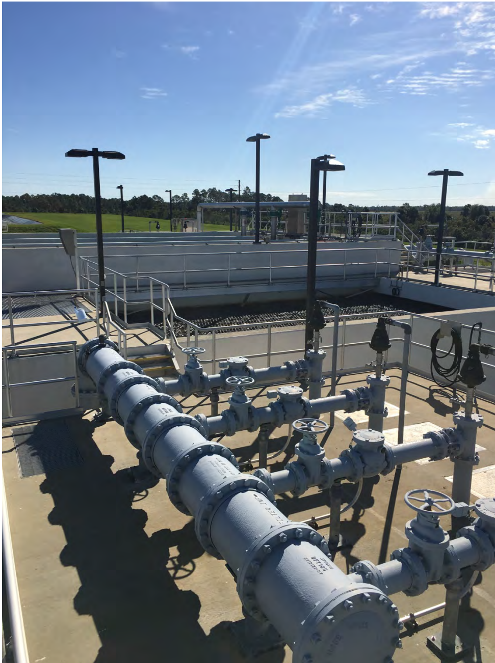
Figure 5-5 Punta Gorda WWTP – Filter Feed Pumps with the Clearwell and Filters in the Background
