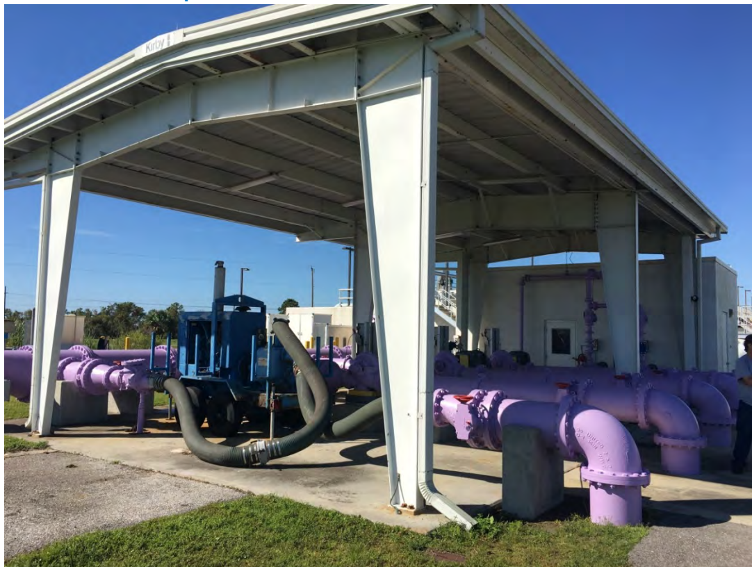
Figure 5-7 Punta Gorda WWTP – Injection Well Pumps and Diesel-Powered Pump
