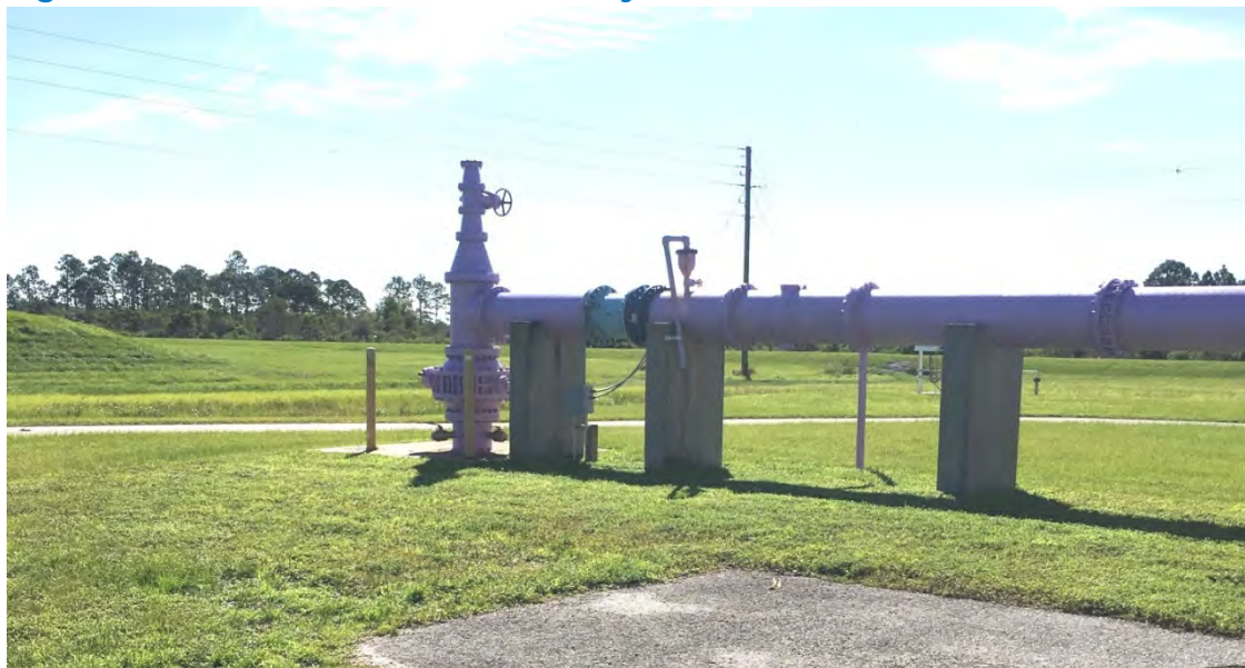
Figure 5-6 Punta Gorda WWTP – Injection Wellhead
