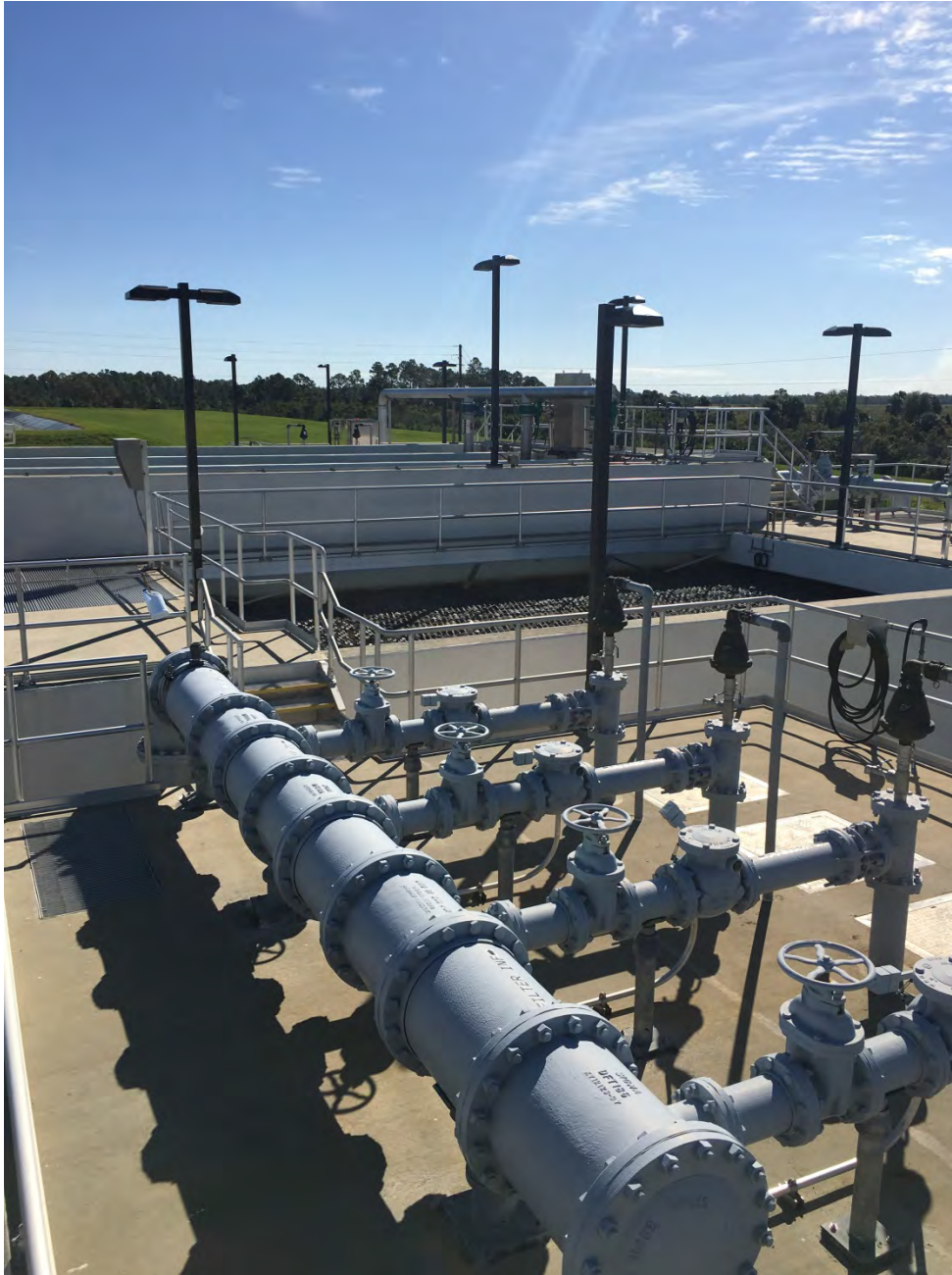
Figure 5-5 Punta Gorda WWTP – Filter Feed Pumps with the Clearwell and Filters in the Background
